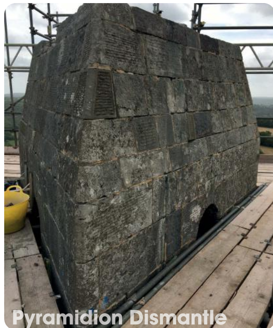
Damage to Walls
